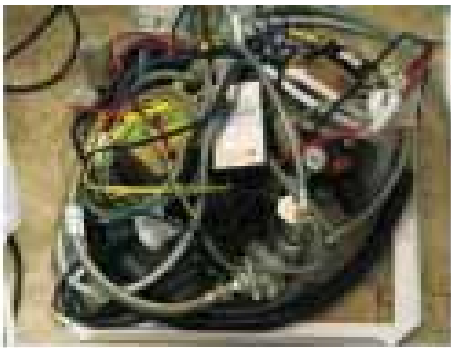
The dental water system is like a maze with about 60 feet of small bore plastic lines with stagnant water for over 20 hours per day in a hot building condition.
